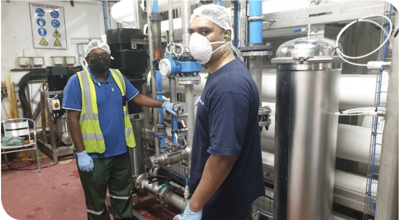
Tyrone Iyavoo (Plant Supervisor) and Avishkar Ramsuren (Process Operator) next to new RO module at CCBSA Premier plant
